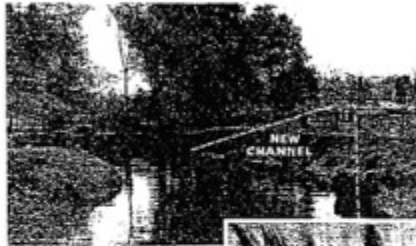
Straightening of Pecon River in New Jersey by CCC workers stopped its yearly floods. Excavation of site indicated to work on right. Start temporary dam at left to provide volume of water for scoring blasted channel.
