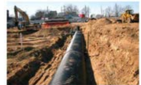
Underground system at Mid Towne Village, Grand Rapids, MI Source: Driesenga & Associates, Inc.
